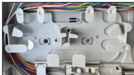
Coiling area for tubes or cables
